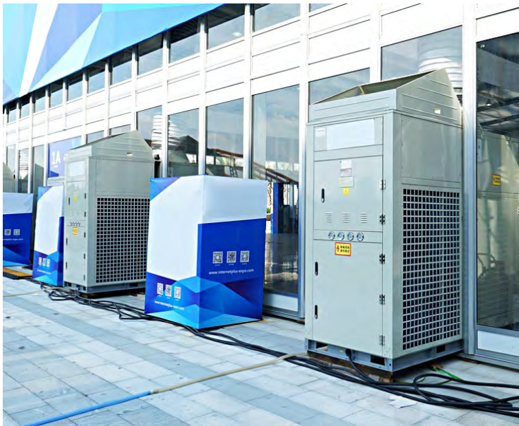
installed partly outside
